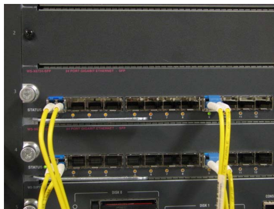
Figure 6: Some Examples of LASER Labels Found in the Verizon Network
